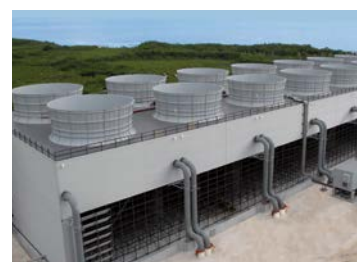
Cooling tower installations
