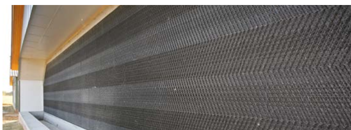
Exhaust air cleaning with NET 150
