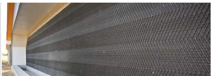
Exhaust air cleaning with 2H NET 150
